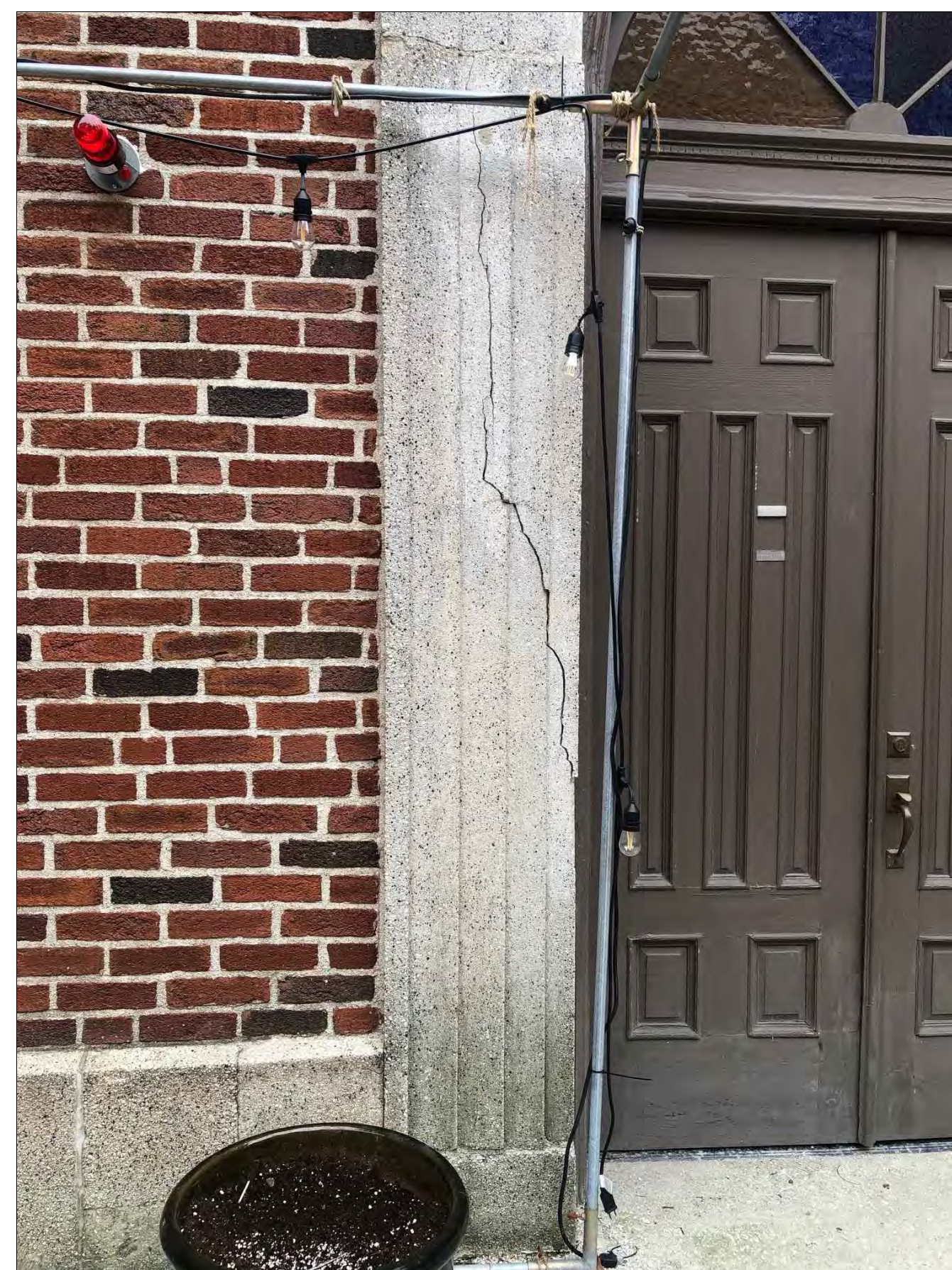
2 CRACKED STONE @LEFT JAMB OVERALL VIEW OF CRACKED PRECAST STONE AT EAST JAMB
