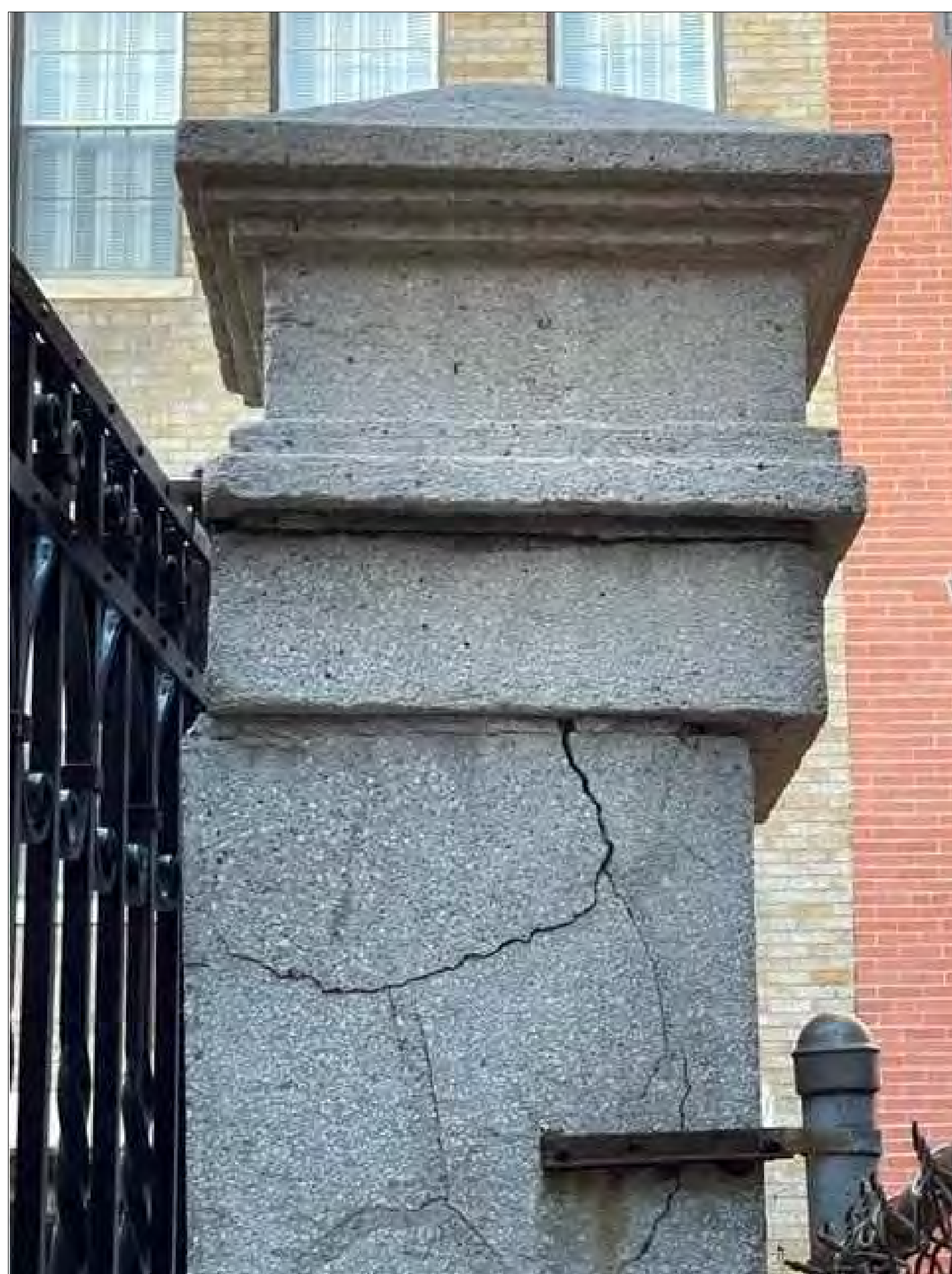
1 CLOSE-UP OF UPPER SOUTH SIDE OF PIER 'A' THIS IS WHERE SAMPLES WERE TAKEN; SEE SHEET A-10.
