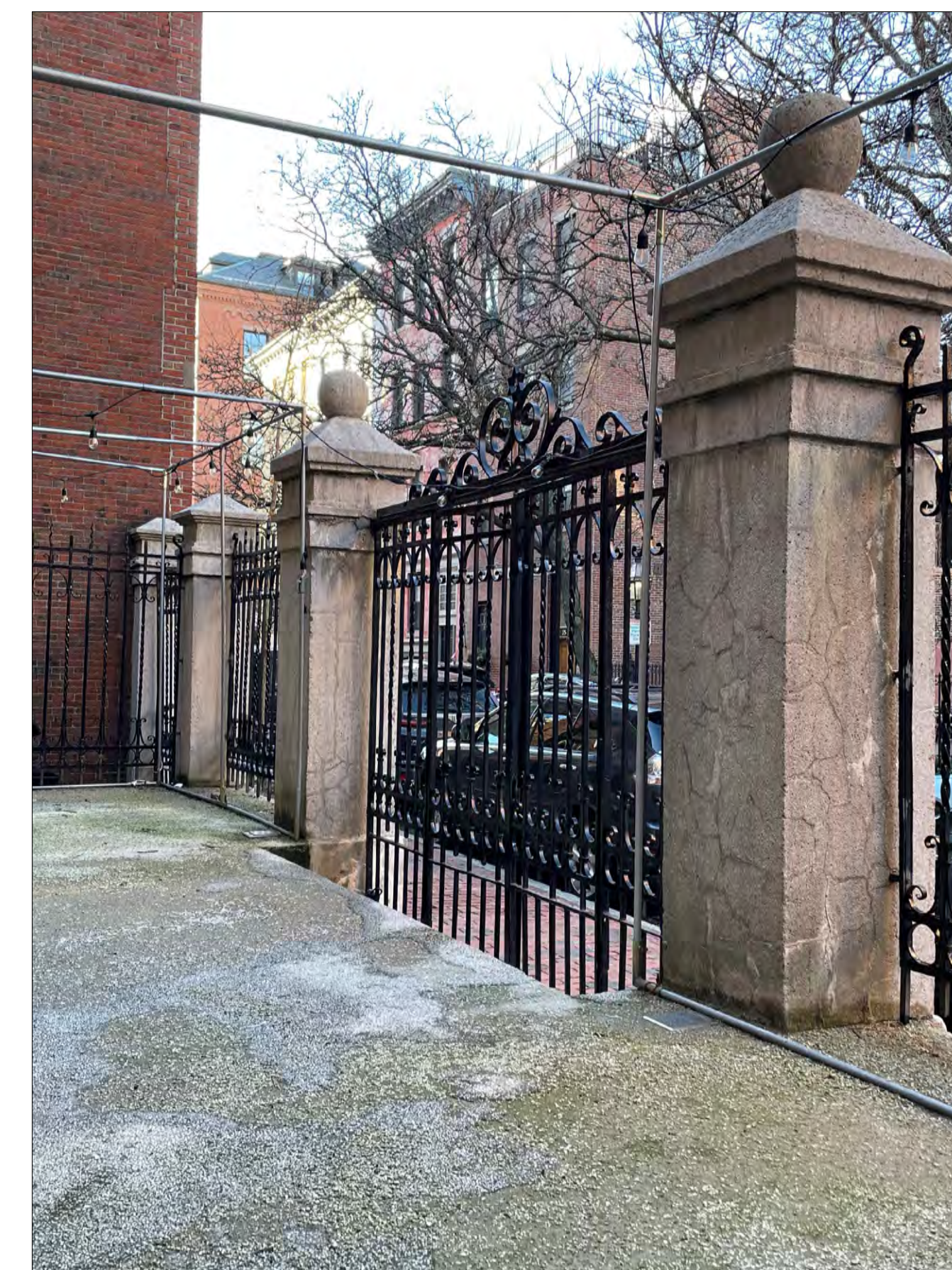
4 EXISTING PLAZA EXISTING DECK CONDITIONS AT ENTRY STAIR AND ENTRY GATES LOOKING TOWARD PHILLIPS STREET SIDEWALK
