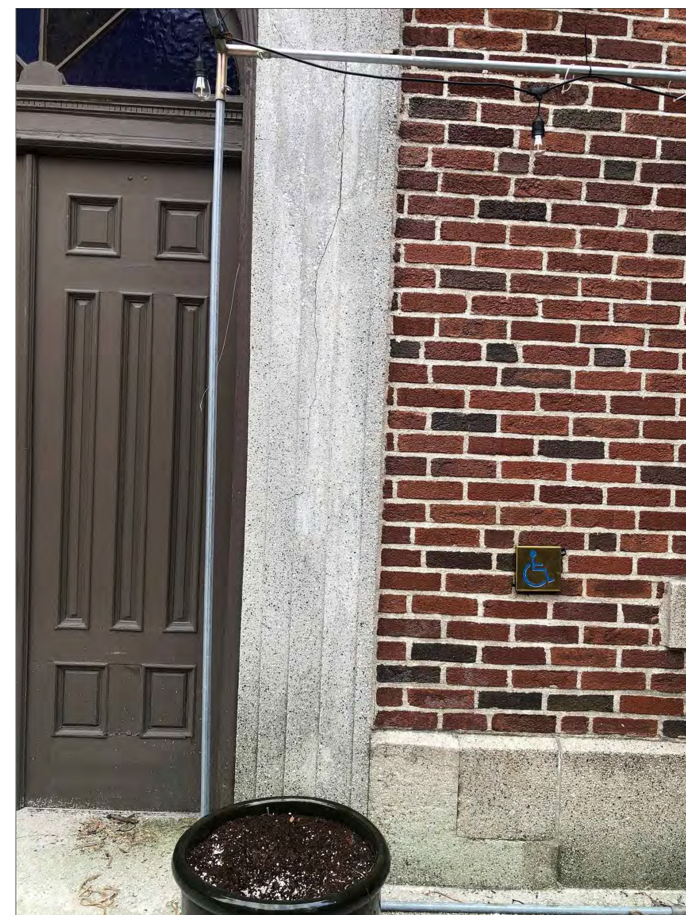
3 CRACKED STONE @ RIGHT JAMB OVERALL VIEW OF CRACKED PRECAST STONE AT WEST JAMB
