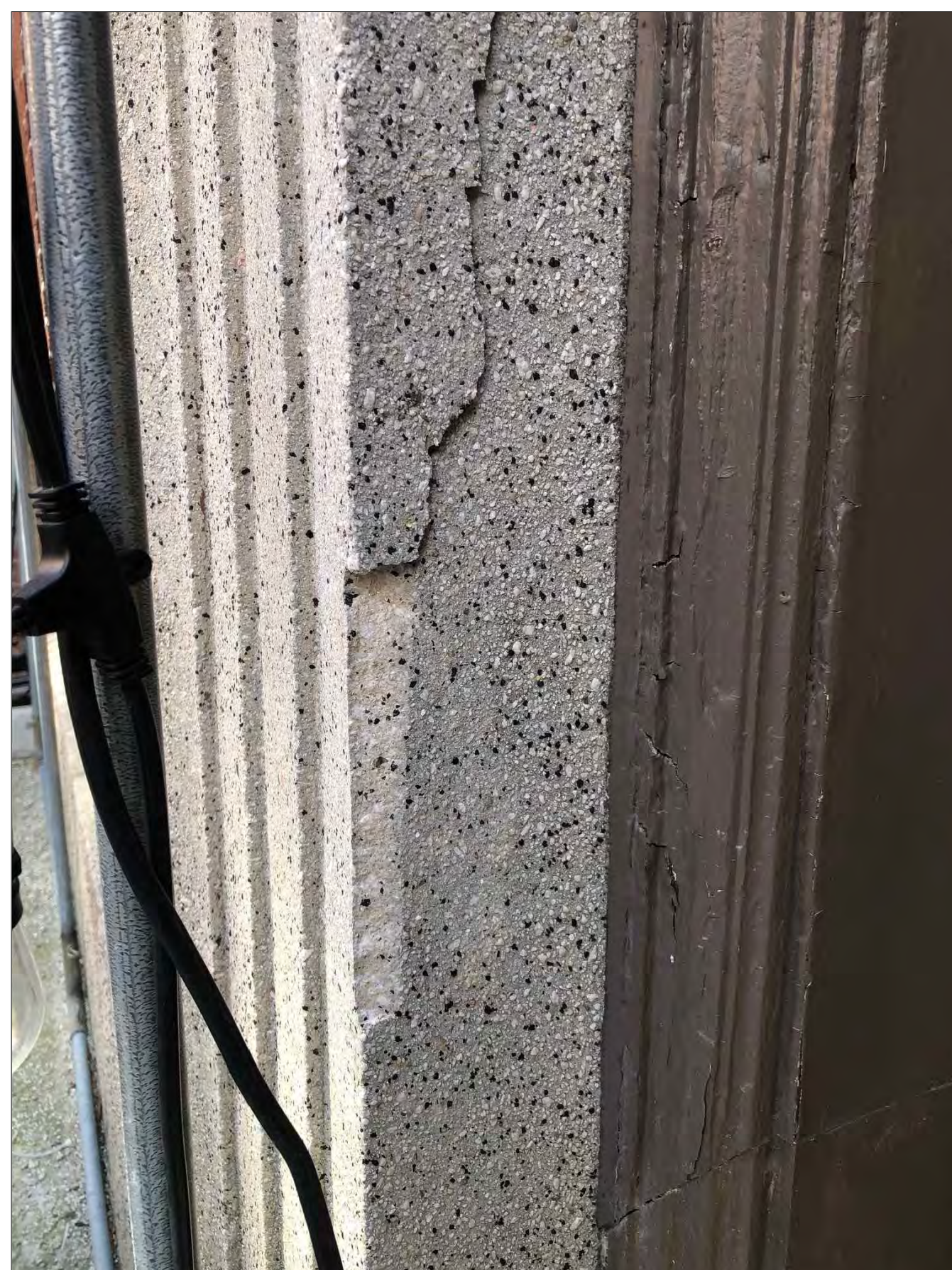
1 CRACKED STONE @LEFT JAMB CLOSE UP OF CRACKED PRECAST STONE AT EAST JAMB
