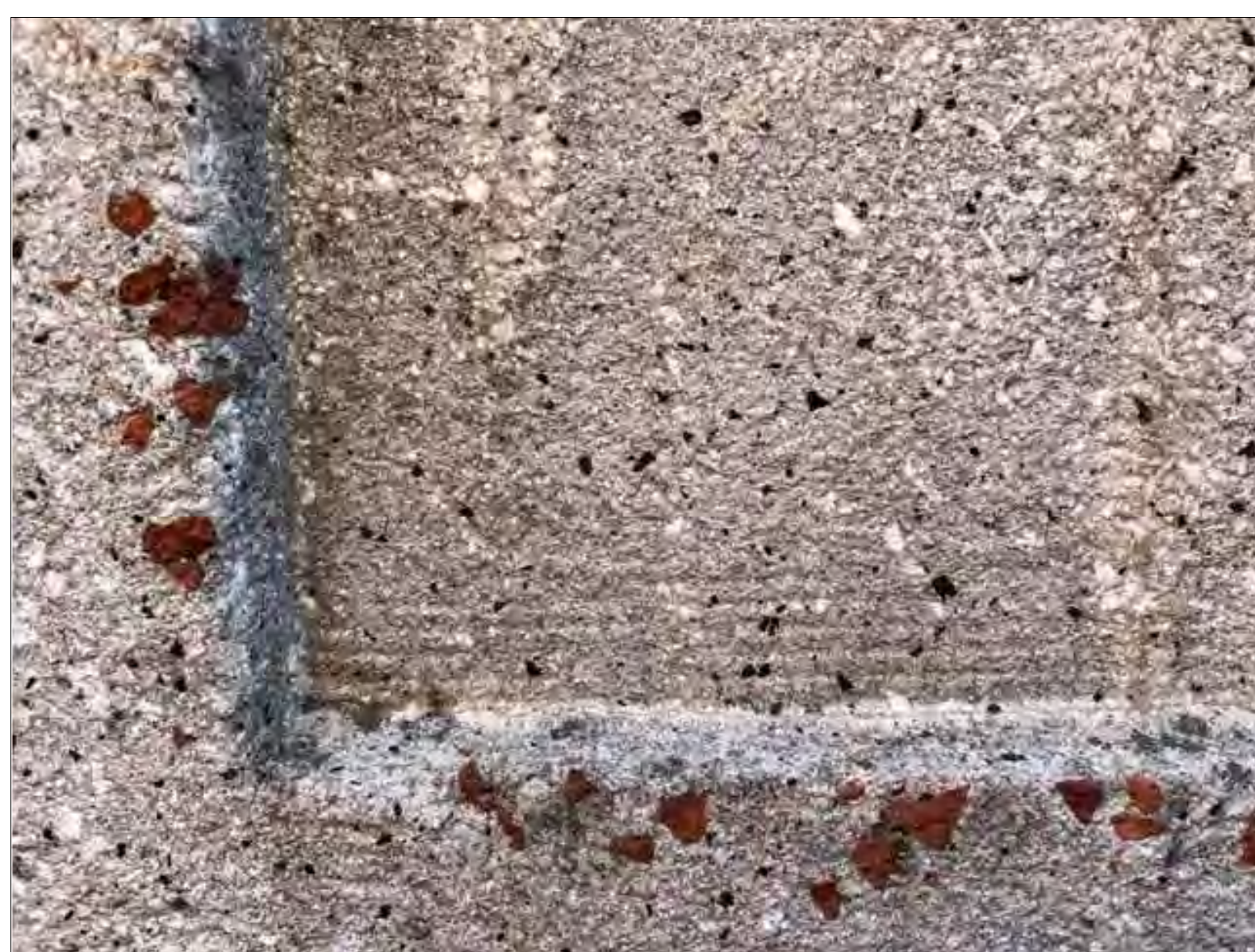
4 CLOSE-UP OF PIER 'B' SHOWING LARGE AGGREGATE NOTICE EVIDENCE OF SURFACE HAVING BEEN WORKED BY BUSH HAMMERS AND PATENT HAMMERS.
