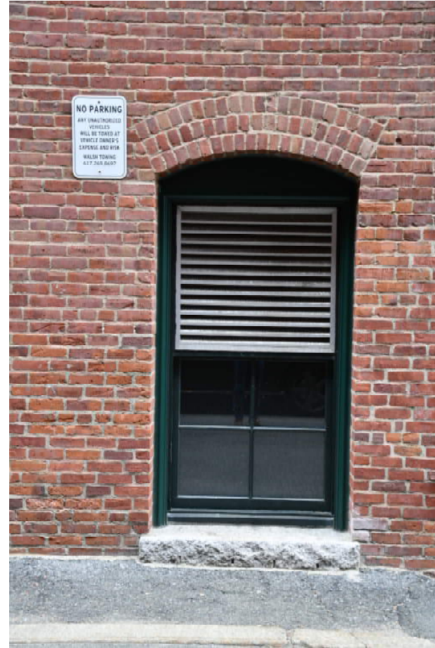
Aluminum window panning trim installed over original wood trim; Window mockup later Rejected and determined that custom trim needs to be made.
