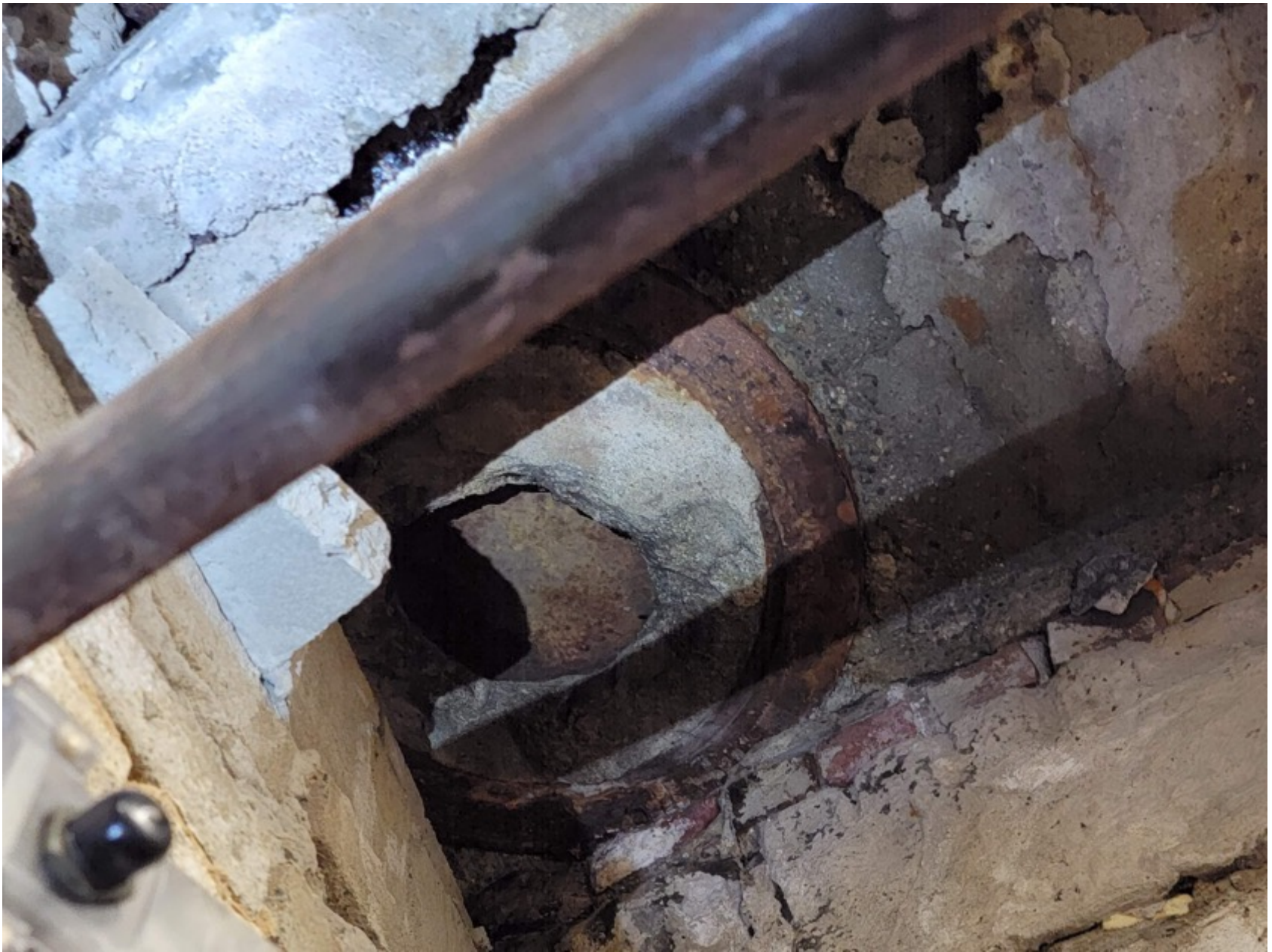
34.5 Beacon Street, Boston, Damage to concrete under the sidewalk in interior space.
