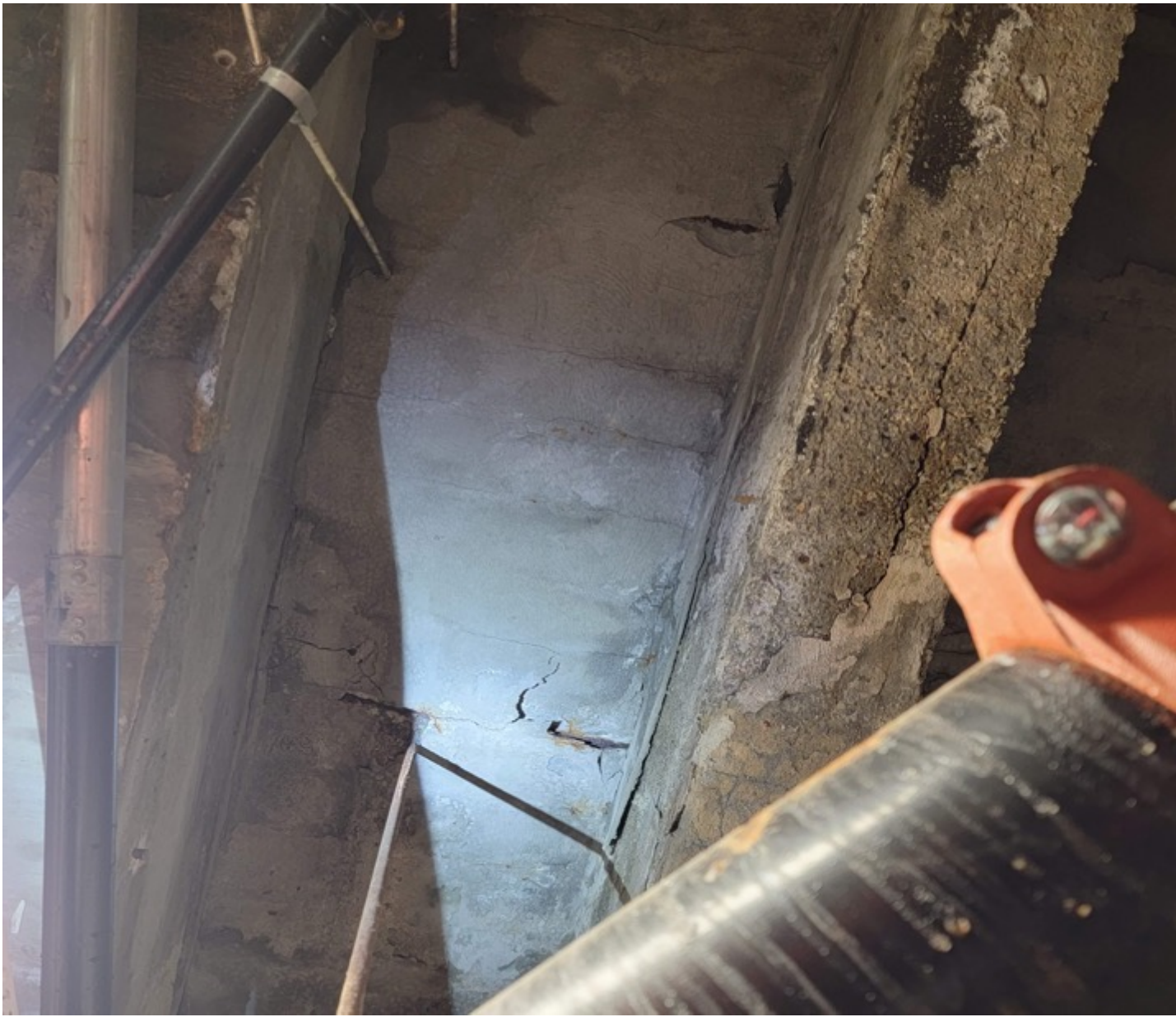
34.5 Beacon Street, Boston, Damage to concrete under the sidewalk in interior space.
