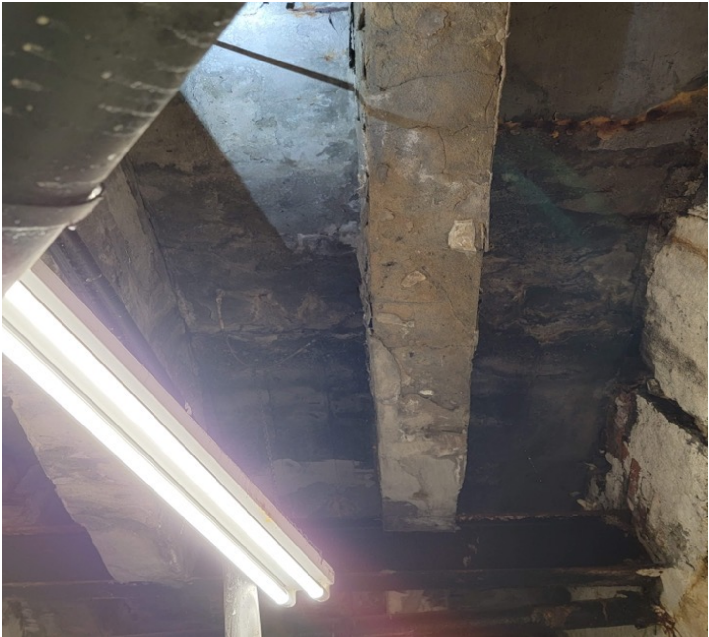
34.5 Beacon Street, Boston, Damage to concrete under the sidewalk in interior space.
