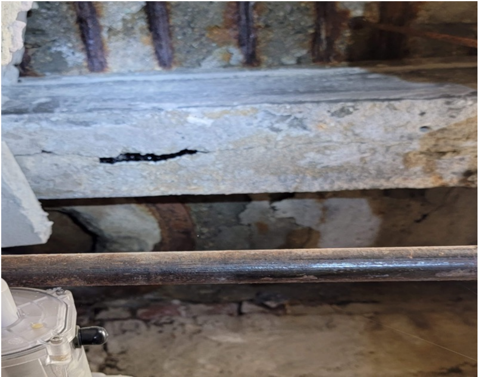
34.5 Beacon Street, Boston, Damage to concrete under the sidewalk in interior space.
