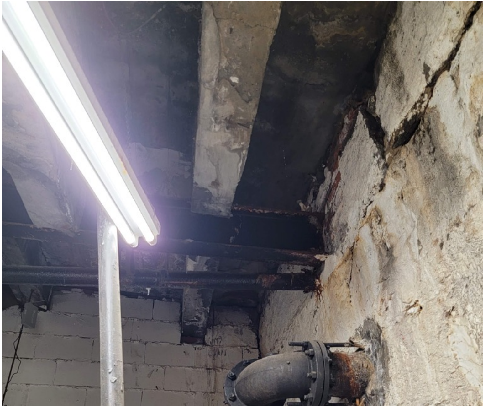
34.5 Beacon Street, Boston, Damage to concrete under the sidewalk in interior space.
