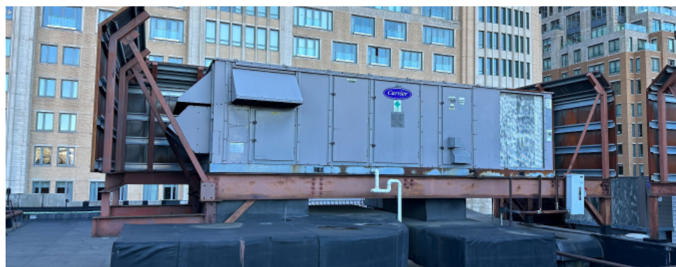
EXISTING ROOFTOP UNIT
