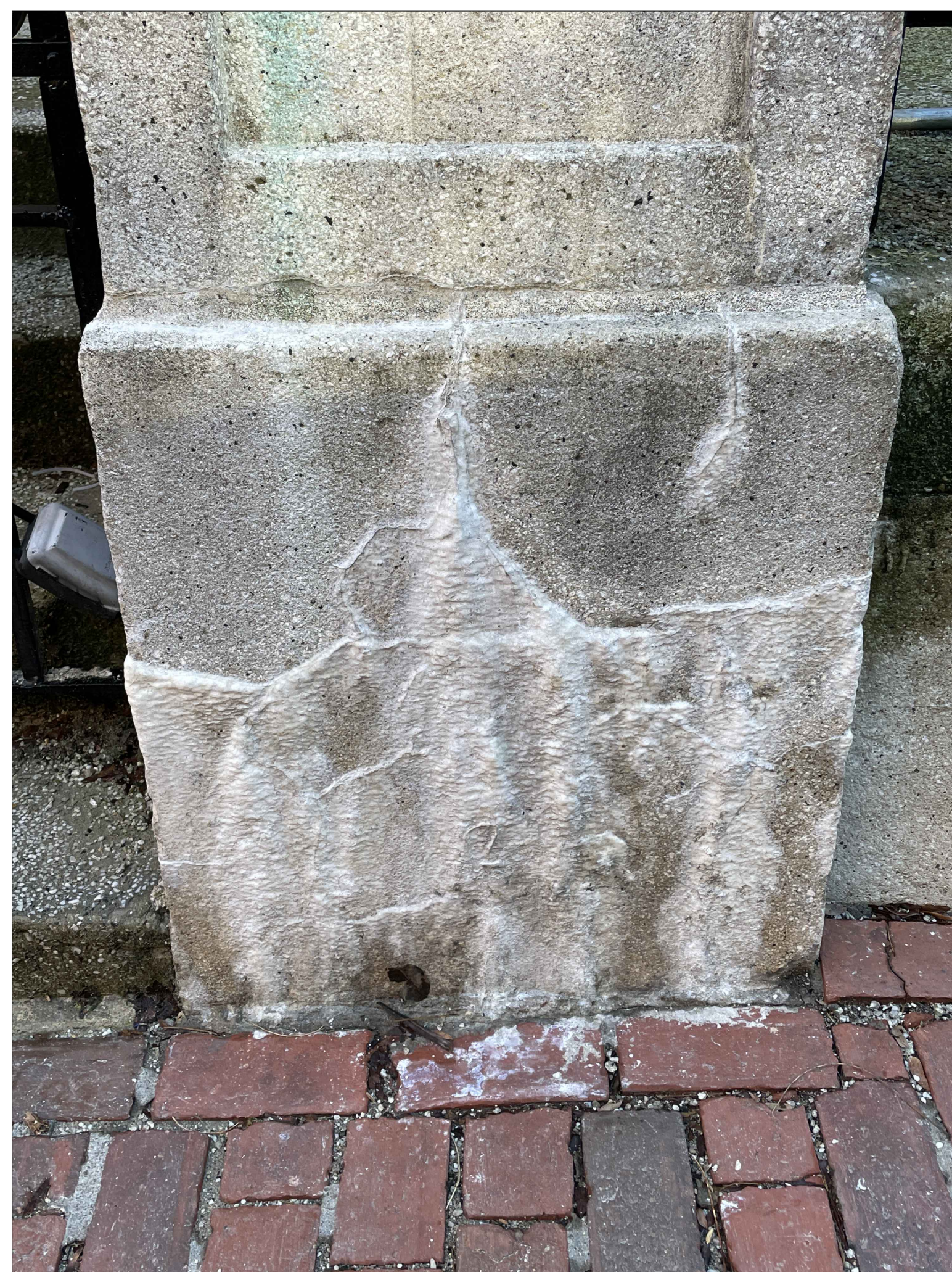
2 SURFACE EFFLORESCENCE AT NORTH SIDE BASE OF PIER 'D'
