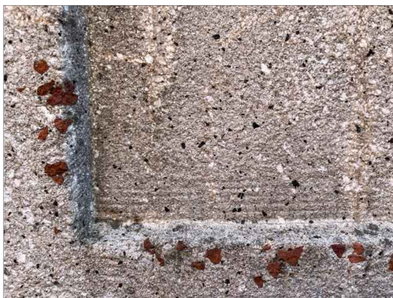
4 CLOSE-UP OF PIER 'B' SHOWING LARGE AGGREGATE NOTICE EVIDENCE OF SURFACE HAVING BEEN WORKED BY BUSH HAMMERS AND PATENT HAMMERS.
