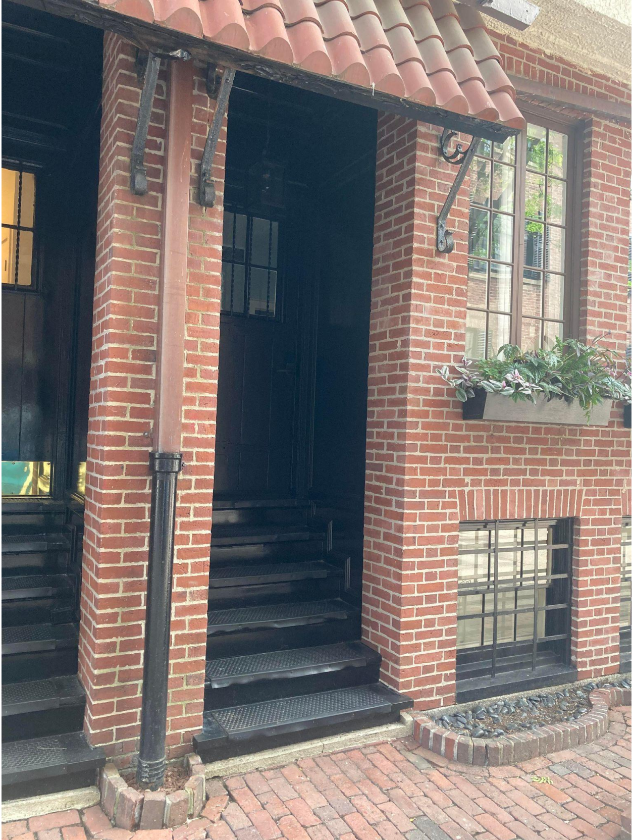
Door between 26 and 30 Lime where the proposed railing is to be installed
