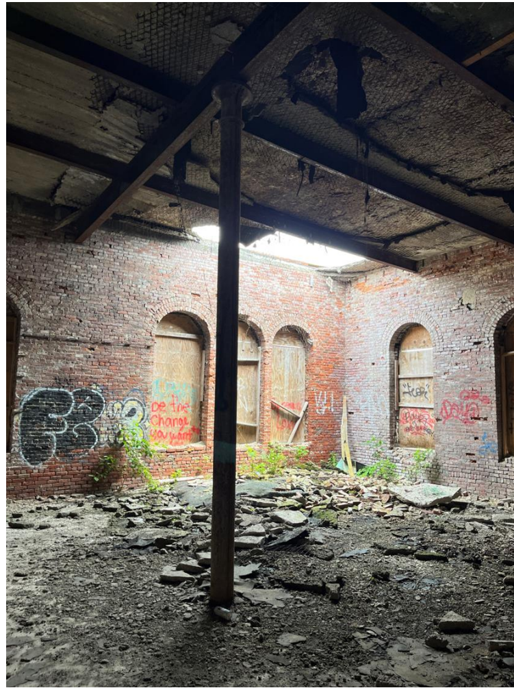
Area of Collapse by Sidewalk
