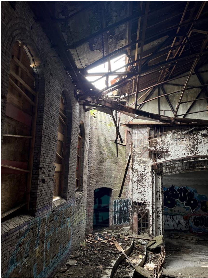
Collapse by Stands
