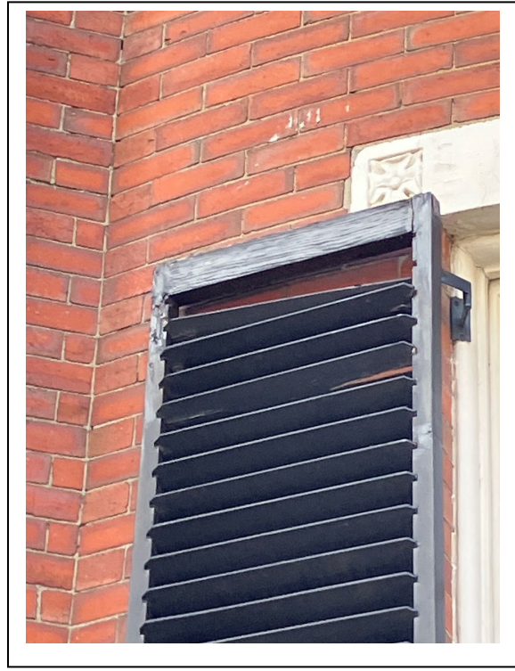
Close up of broken & worn shutter to be replaced
