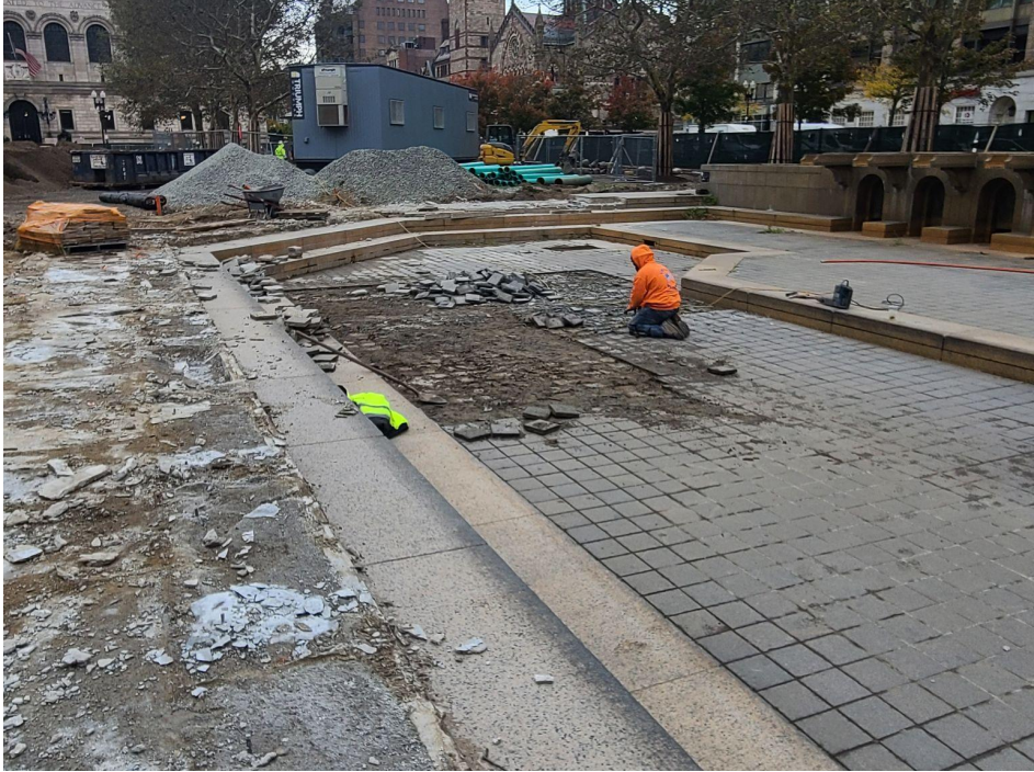
Hand removal of the fountain basin tiles will allow us to reuse those in good condition.
