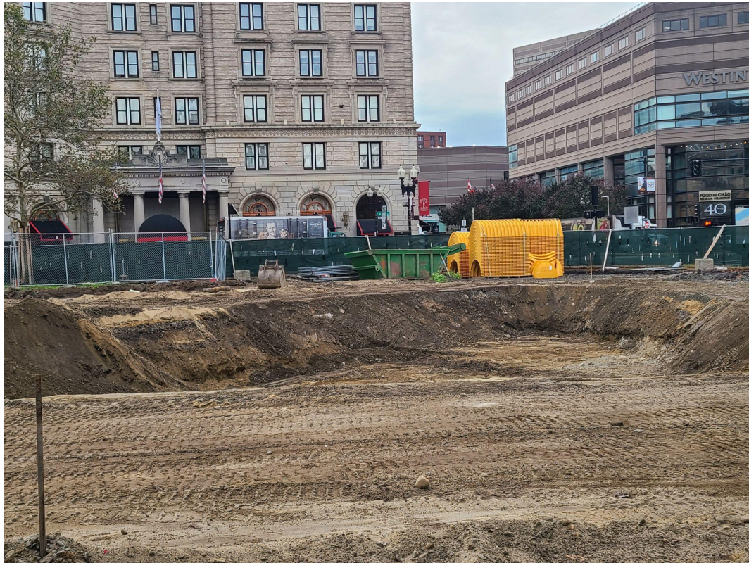
The excavation area for the infiltration chamber: Pieces of the chamber were just delivered to the site - the bright yellow material on the far side of the pit. (That's not play equipment!)
