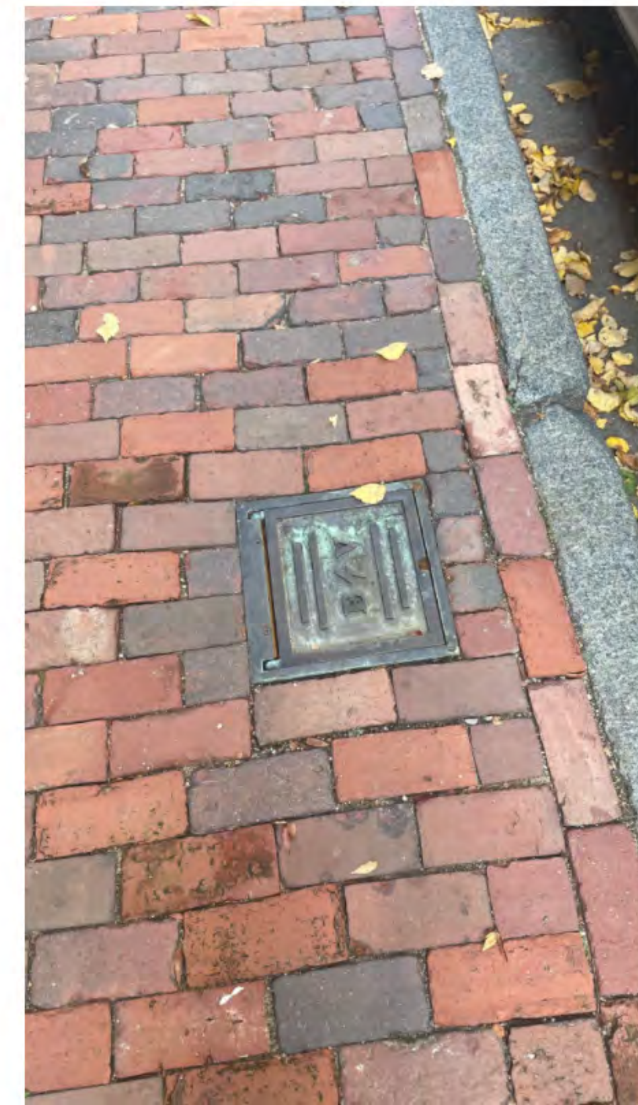
SIMILAR EV CHARGER INSTALLED AT 18 LOUISBURG SQUARE
