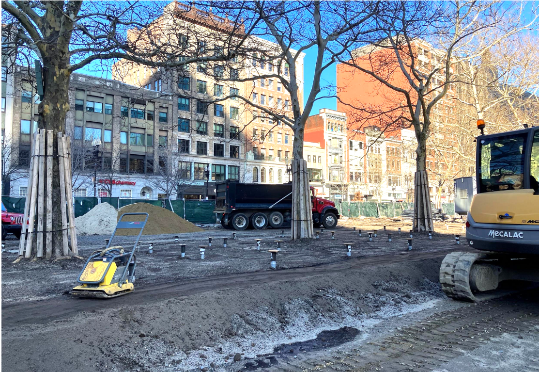
At the Raised Grove, the tops of the piles (pile caps) are just visible, sticking up above the planting soil. The grade beam will rest on top of the piles, and the planks of the surface will rest on the grade beam.
