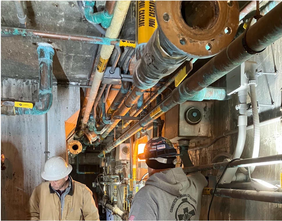
Inside the fountain vault, some pipes remain and many have been removed. We need to waterproof the walls and make sure that sufficient space exists for new vents, new pipes, and new electrical systems.
