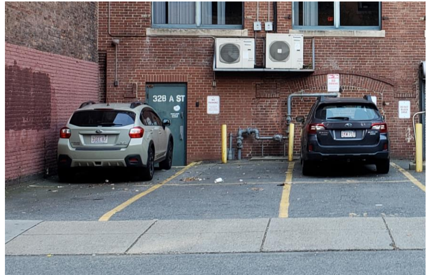
CONDENSERS AT 328 STREET
