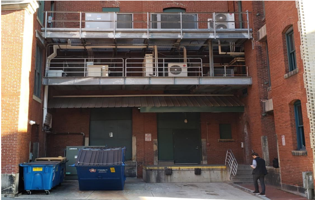
CONDENSERS BEHIND 281-283 SUMMER STREET
