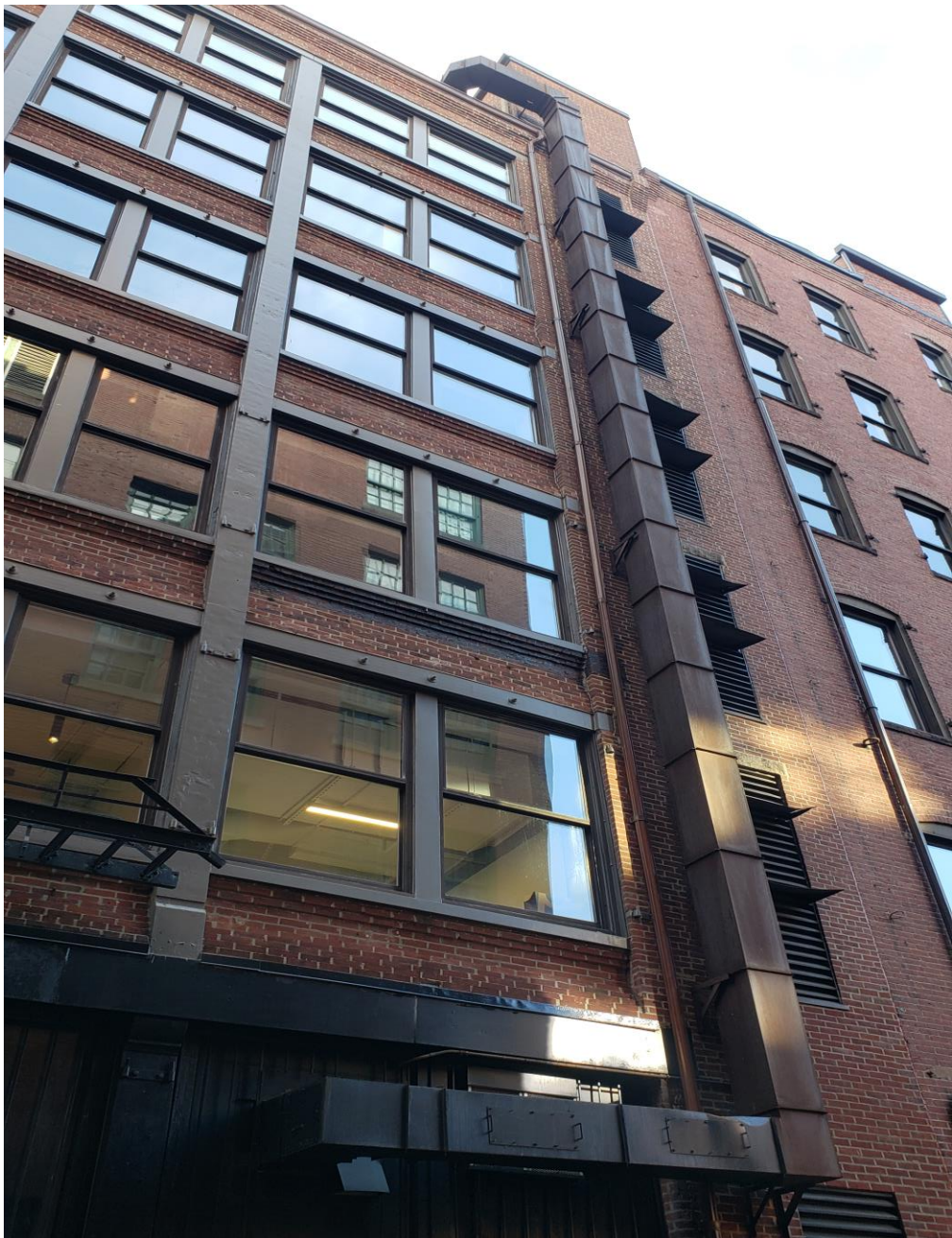
SURFACE MOUNTED DUCTWORK BEHIND "METRO" SPACE
