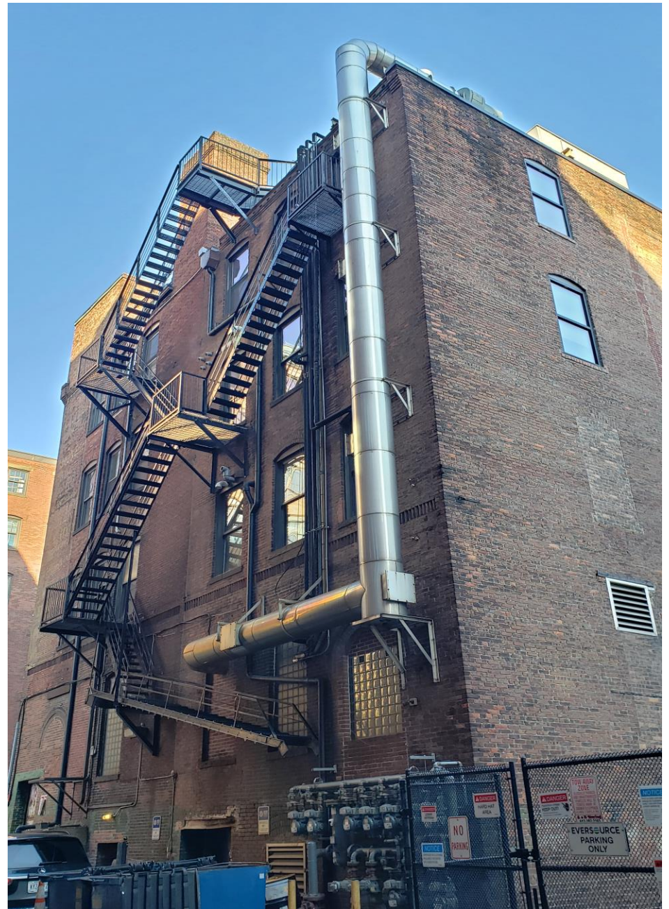
SURFACE MOUNTED DUCTWORK BEHIND "LUCKY'S"
