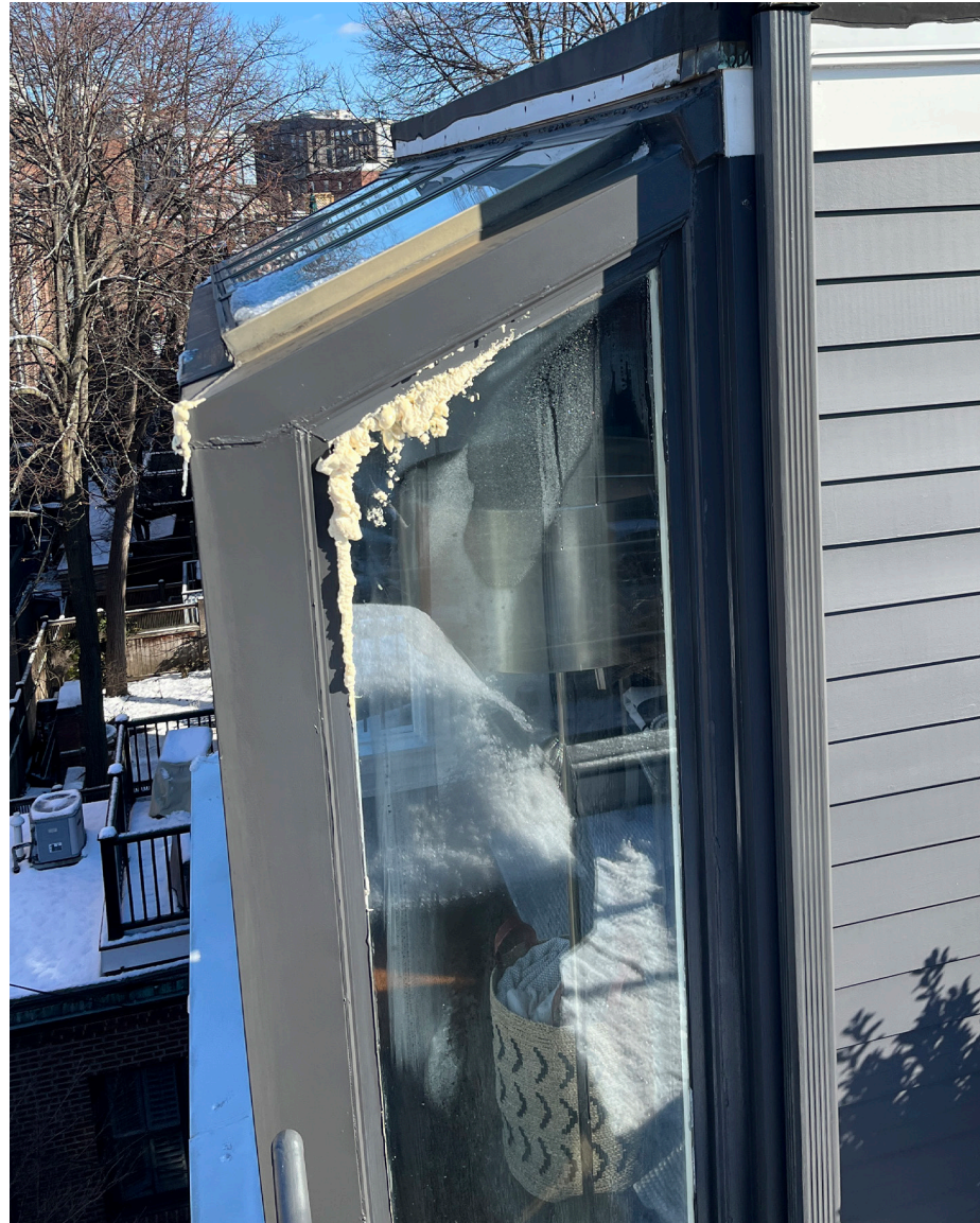
Existing conditions of deteriorated glazed skylight enclosure with failing seals.
