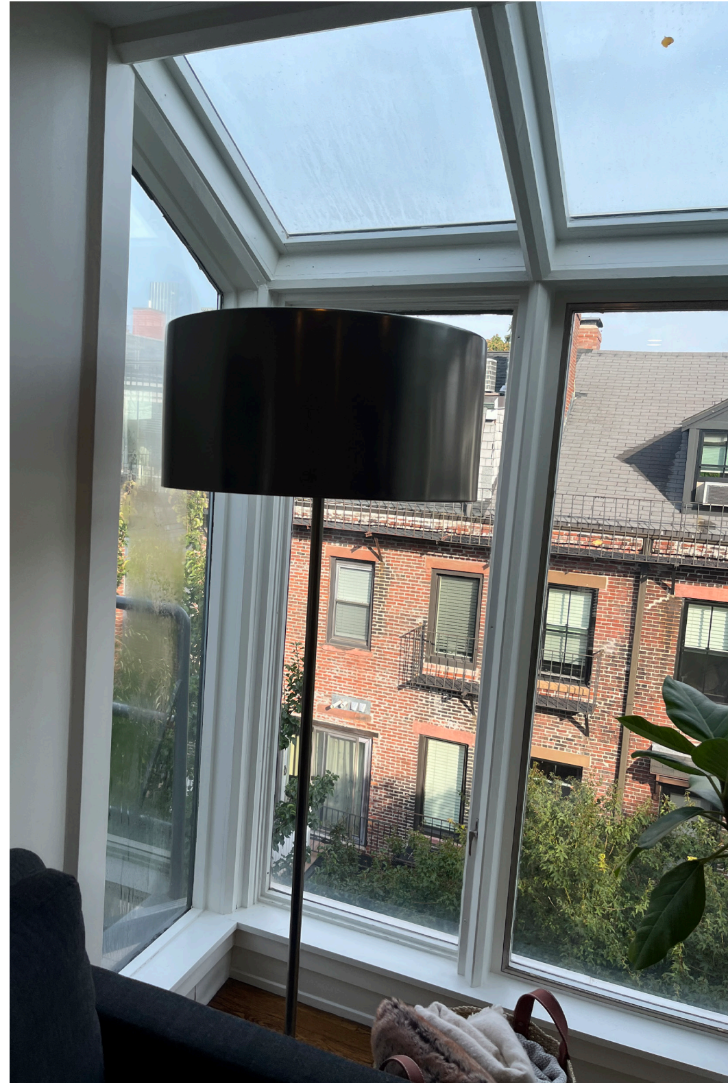
Photo taken from inside of broken seals with condensation in panes.
