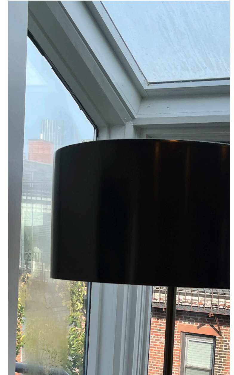
Close up of condensation in panes.
