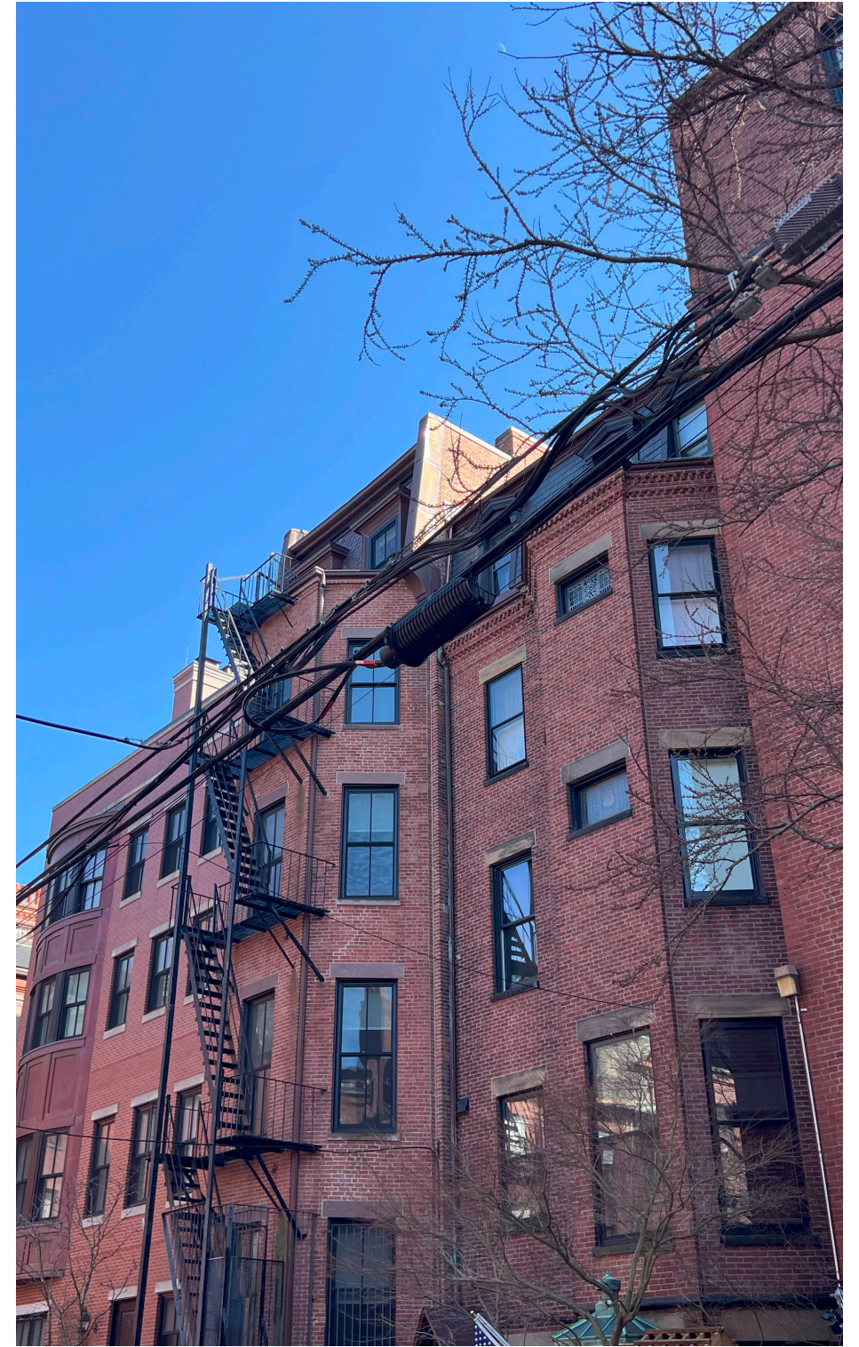
PHOTOS WITH MOCK UP IN PLACE FROM ALLEY 163 COMMONWEALTH AVE 20 MARCH 2024 CATHERINE TRUMAN ARCHITECTS
