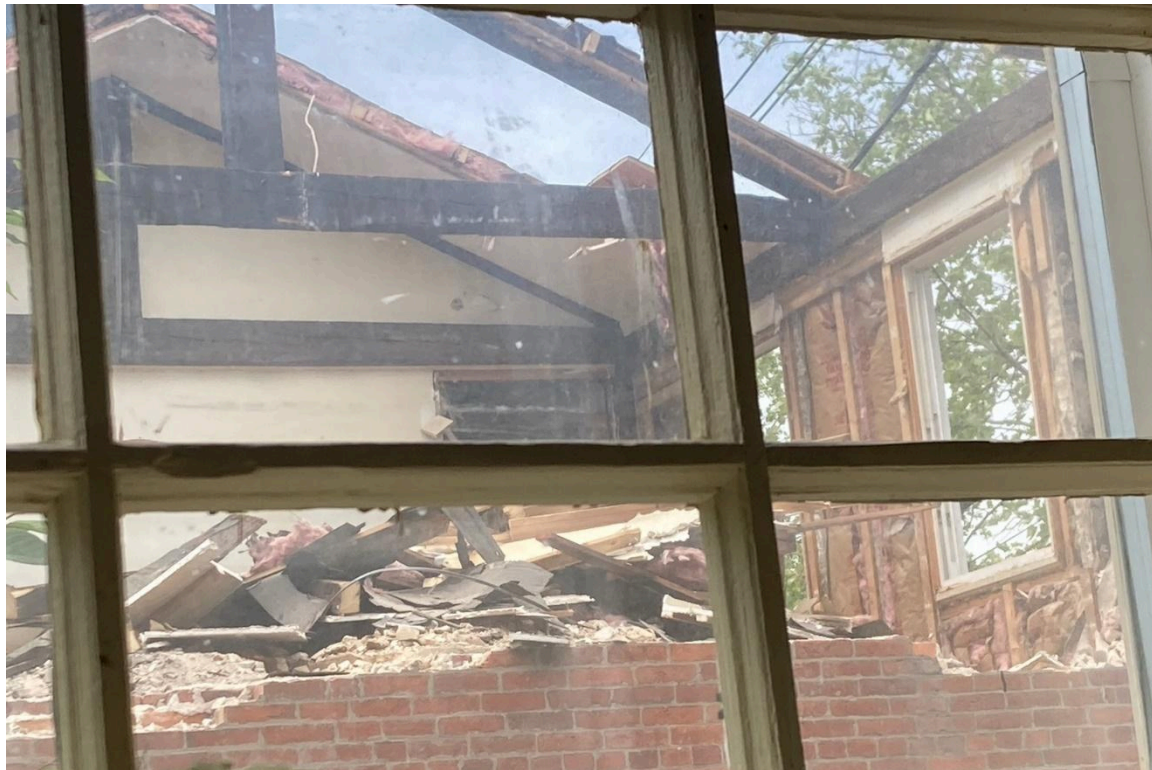
Photo 4. 8 Lawrence Street (May 2022, during demolition), view of roof truss system and second-story rooms, looking north.
