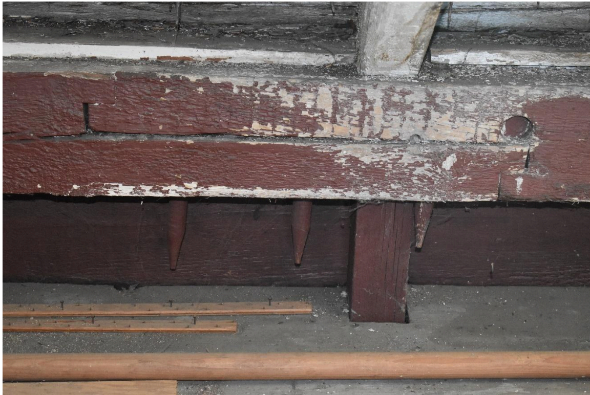
Figure 17. Attic, showing sistered eave plate with dowels, rafter (white), and secondary post (red). Photo by The Public Archaeology Laboratory, Inc.
