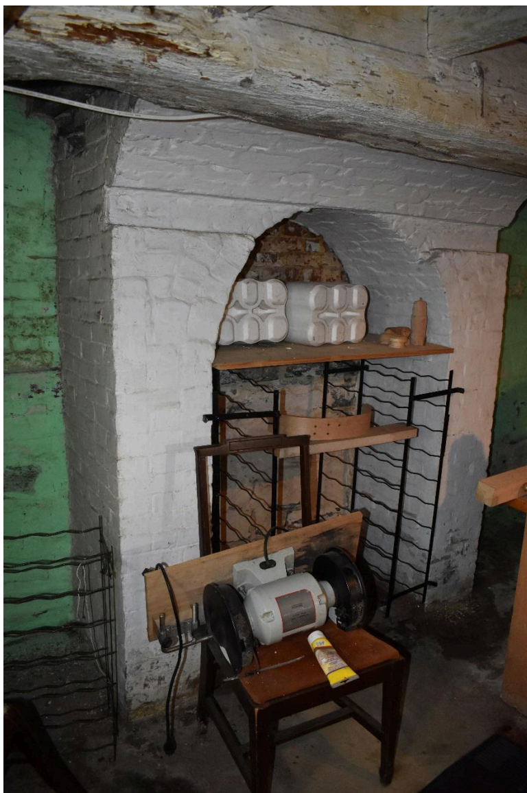
Figure 9. Basement, southwest chimney relieving arch. Photo by The Public Archaeology Laboratory, Inc.
