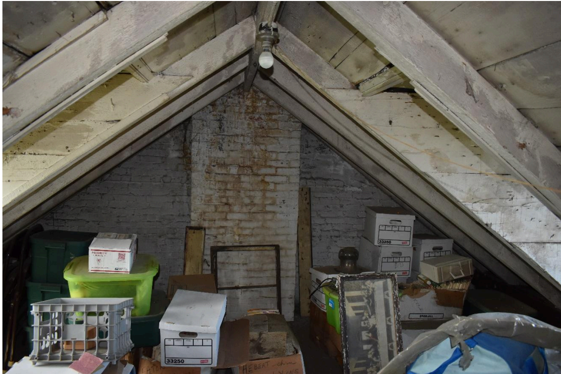
Figure 16. Attic with brick end wall and ridge board, looking southwest. Photo by The Public Archaeology Laboratory, Inc.
