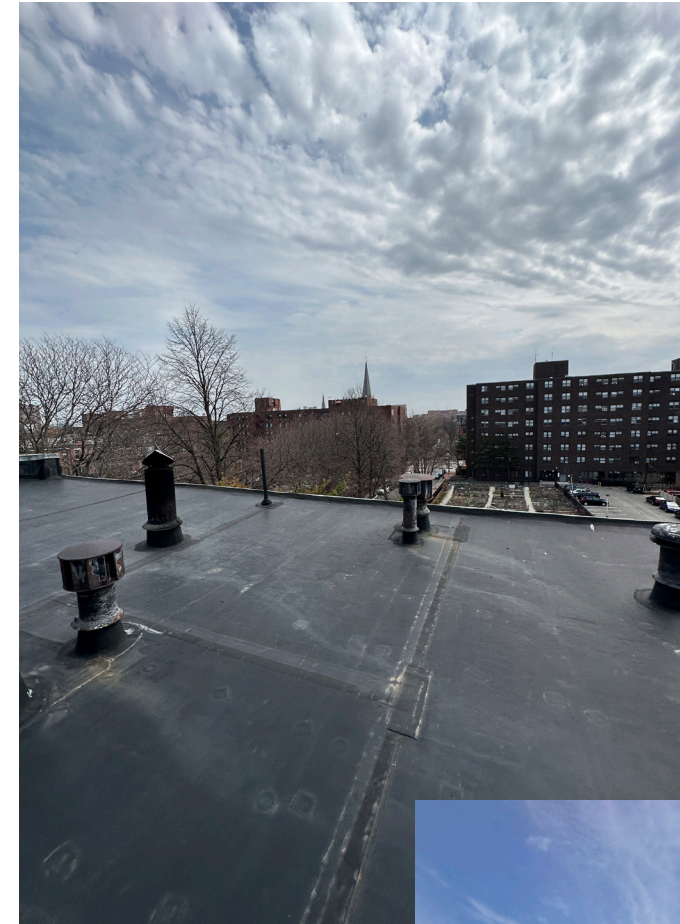
No existing parapet on South elevation. (Community Garden facing facade)
