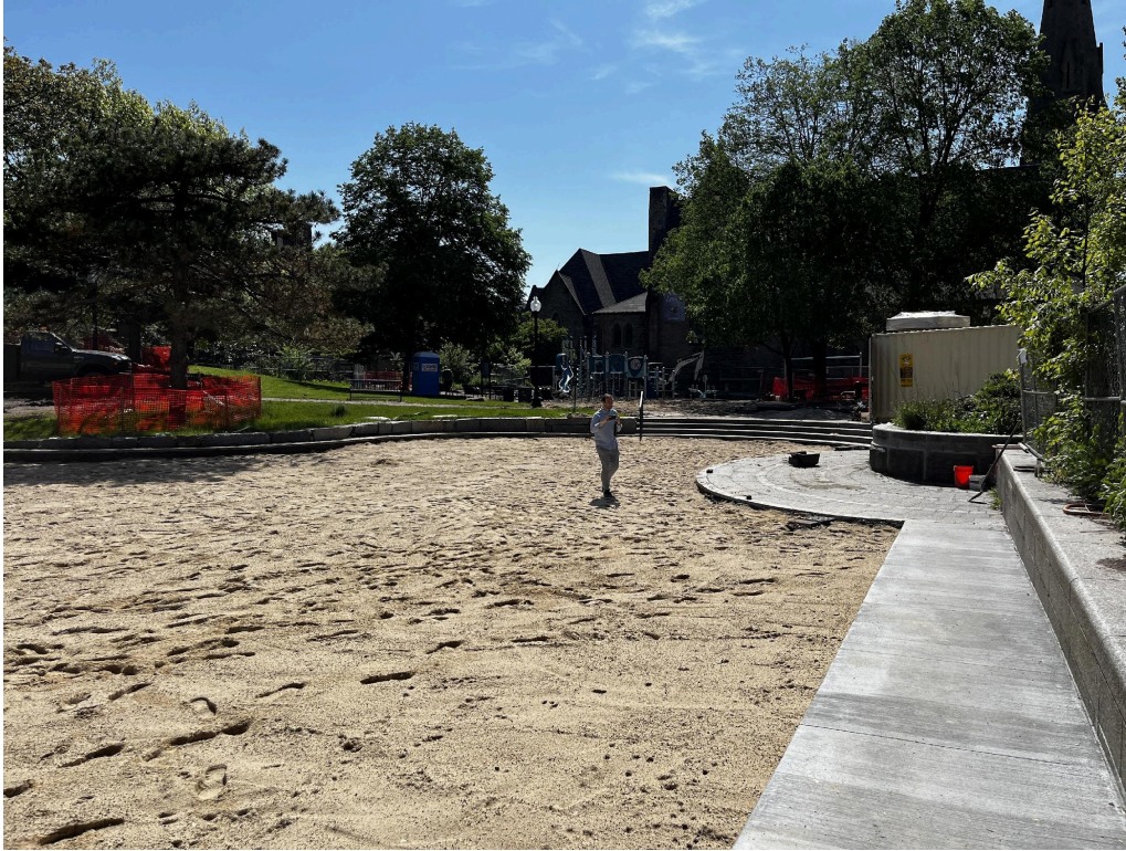
The subsurface drainage system, subgrade, and sand filter layer have been installed SITE PHOTO 5/17/24
