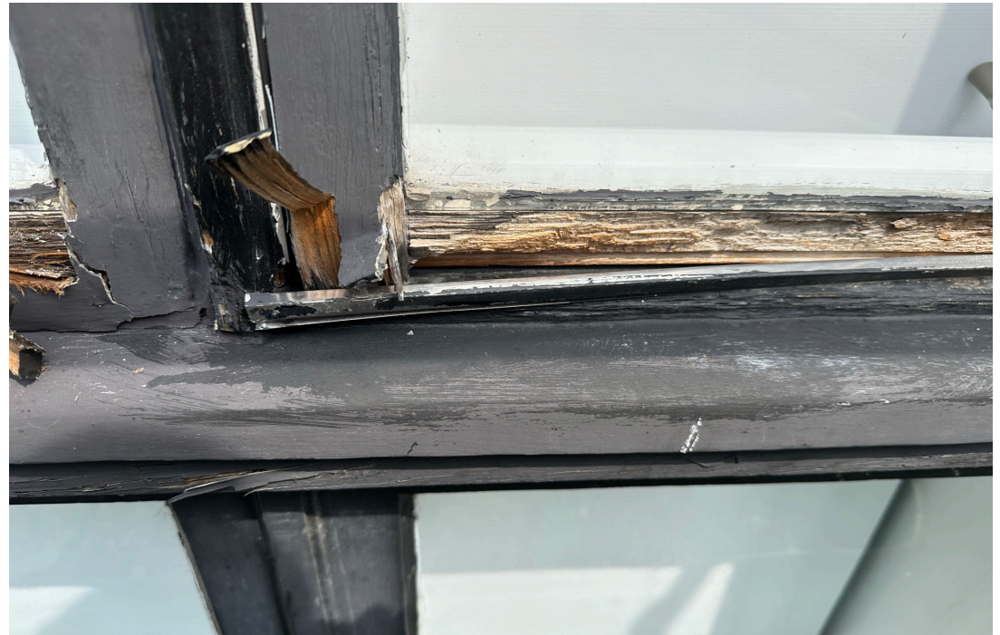
Failed previous repairs
