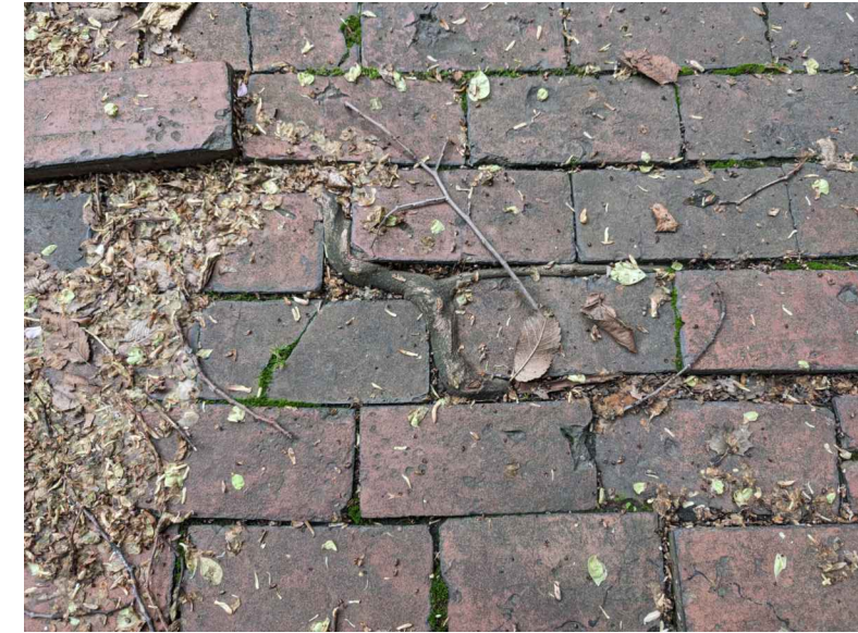
VIEW OF PATIO SHOWING TREE ROOTS BETWEEN PAVERS
