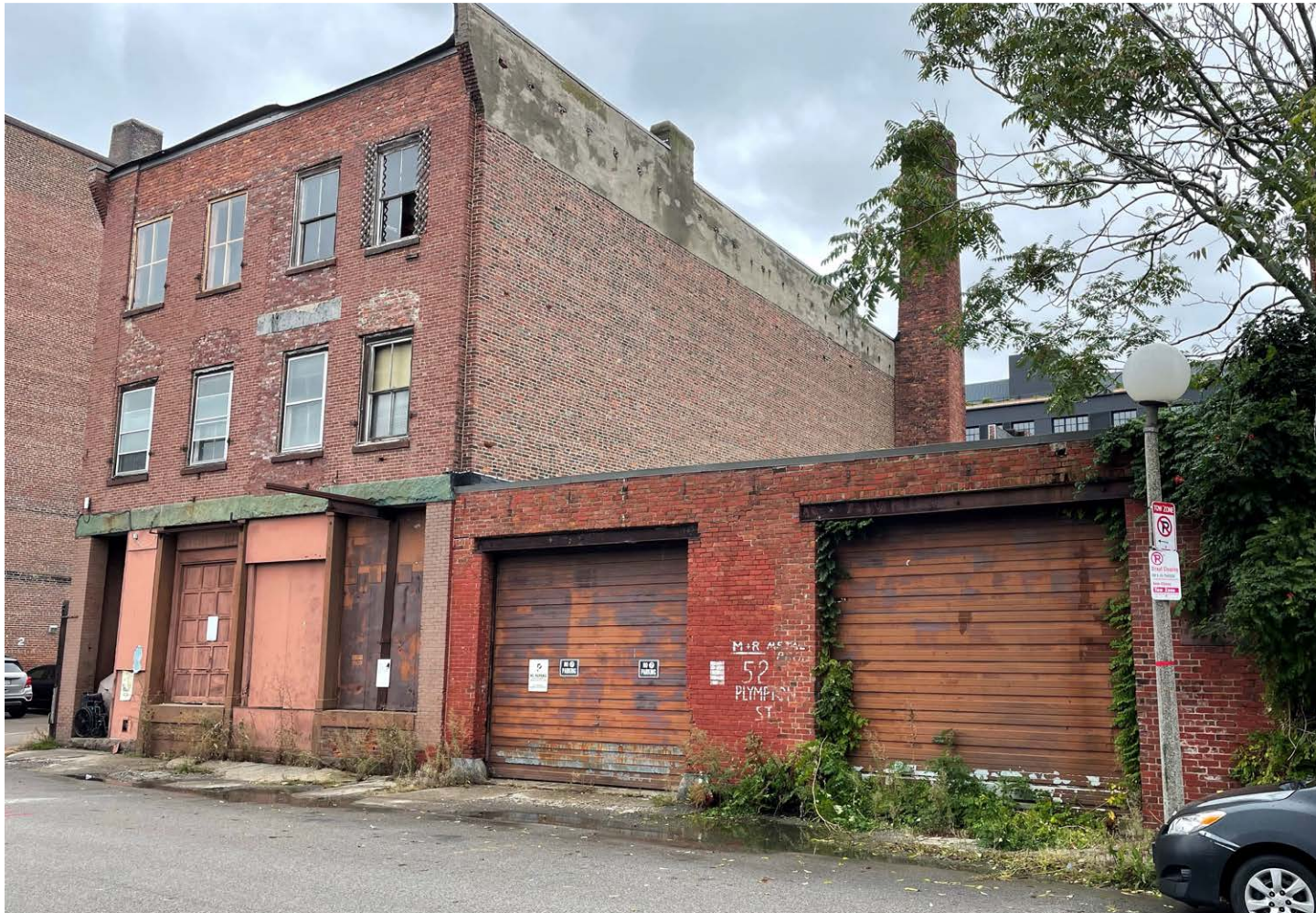
Figure X: Front facade of 52 & 56 Plympton Street. Note the following critical conditions that diminish the building's architectural and structural integrity: The removal of the original historic cornice and the upper-floor window lintels. The conversion of two original storefront bays into loading docks, compromising the structure of the ground floor. Significant masonry deterioration and evidence of settlement across the facade, which has been partially disguised by repointing.
