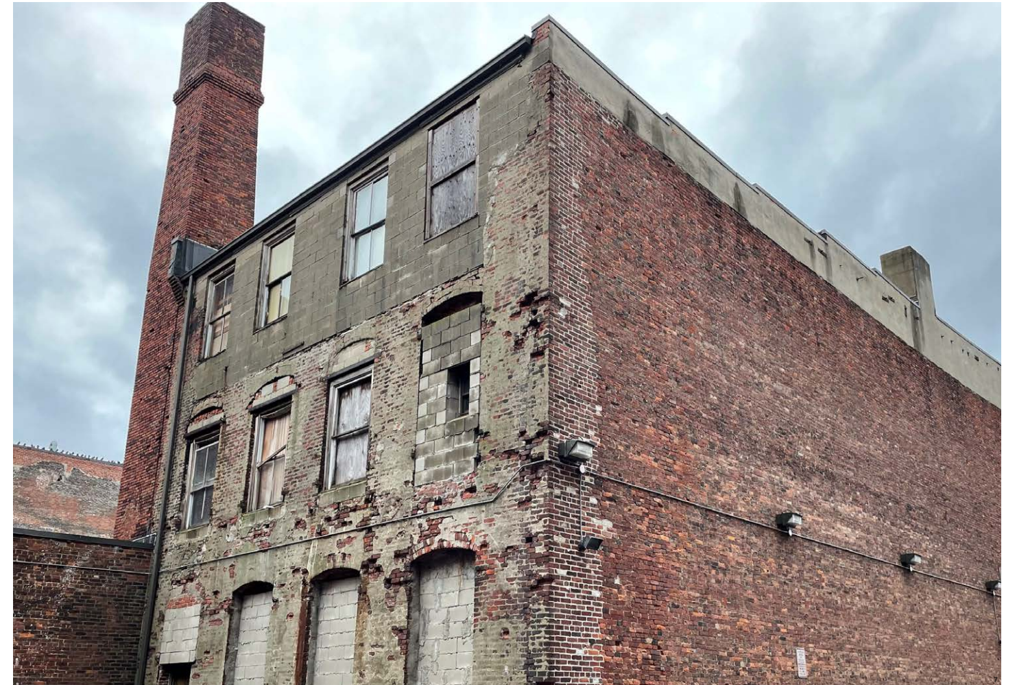
Figure Y: Rear facade of 52 Plympton Street. The rear facade exhibits significant structural issues consistent with the building's overall state of decline. This includes widespread masonry deterioration and evidence of structural settlement. These conditions, which will be further detailed in a forthcoming structural engineering report, contribute to the building's compromised integrity and the infeasibility of its restoration.
