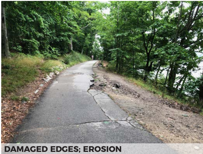
DAMAGED EDGES; EROSION
